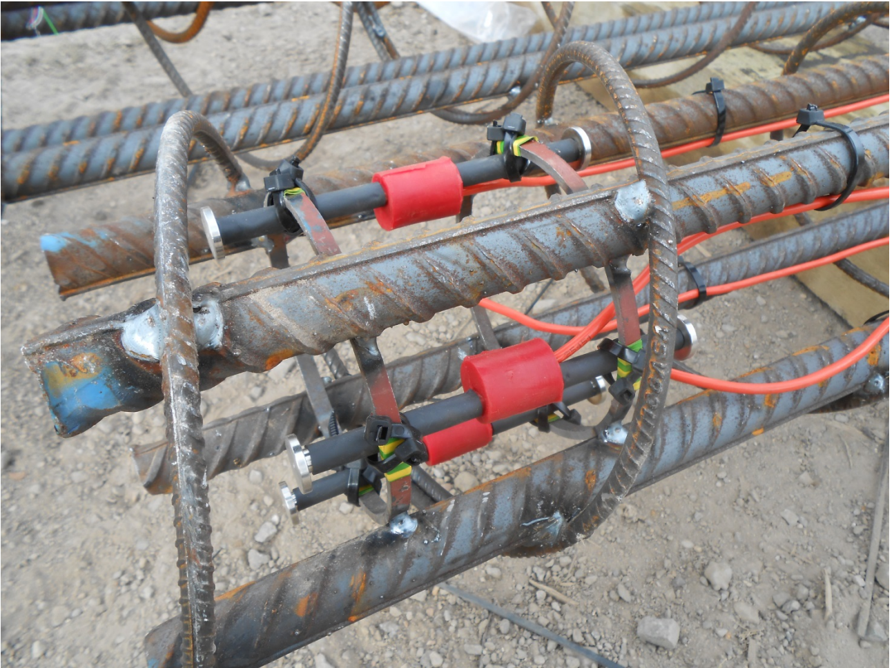
Fig. 6. Arrangement of vibrating wire strain gauge array.
