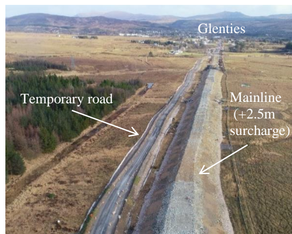
Figure 1. Looking south towards Glenties: temporary diversion on left and main embankment at surcharge level.
