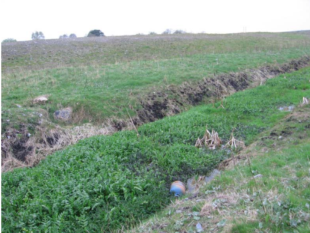
Figure 6 – Clogged stream diversion shown at front and peat disposal area in background at Pollboy 3 years after construction
